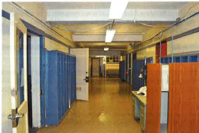
Fig 46. Vinyl asbestos tile in the basement are recommended to be removed.
