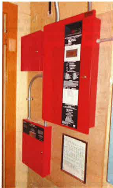
Fig 20. Fire Alarm panel in electrical room in basement.
