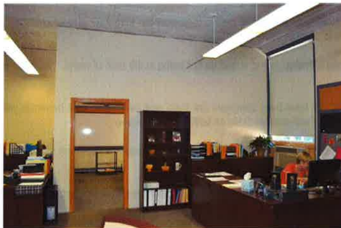
Fig 45. Interior partition recommended to be removed from a third floor classroom.
