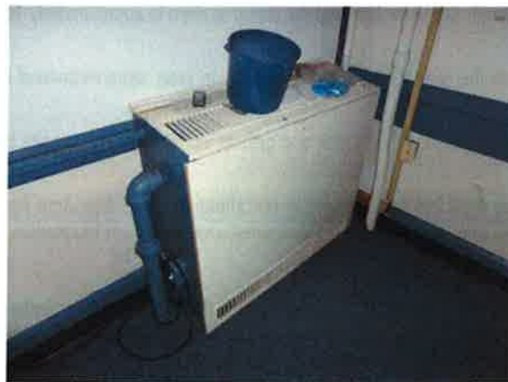
Fig 12. Existing unit ventilator
