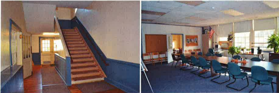
Fig 43. View of metal stair at north entrance. Handrails and a guardrail would be need to bring the stair up to code.
