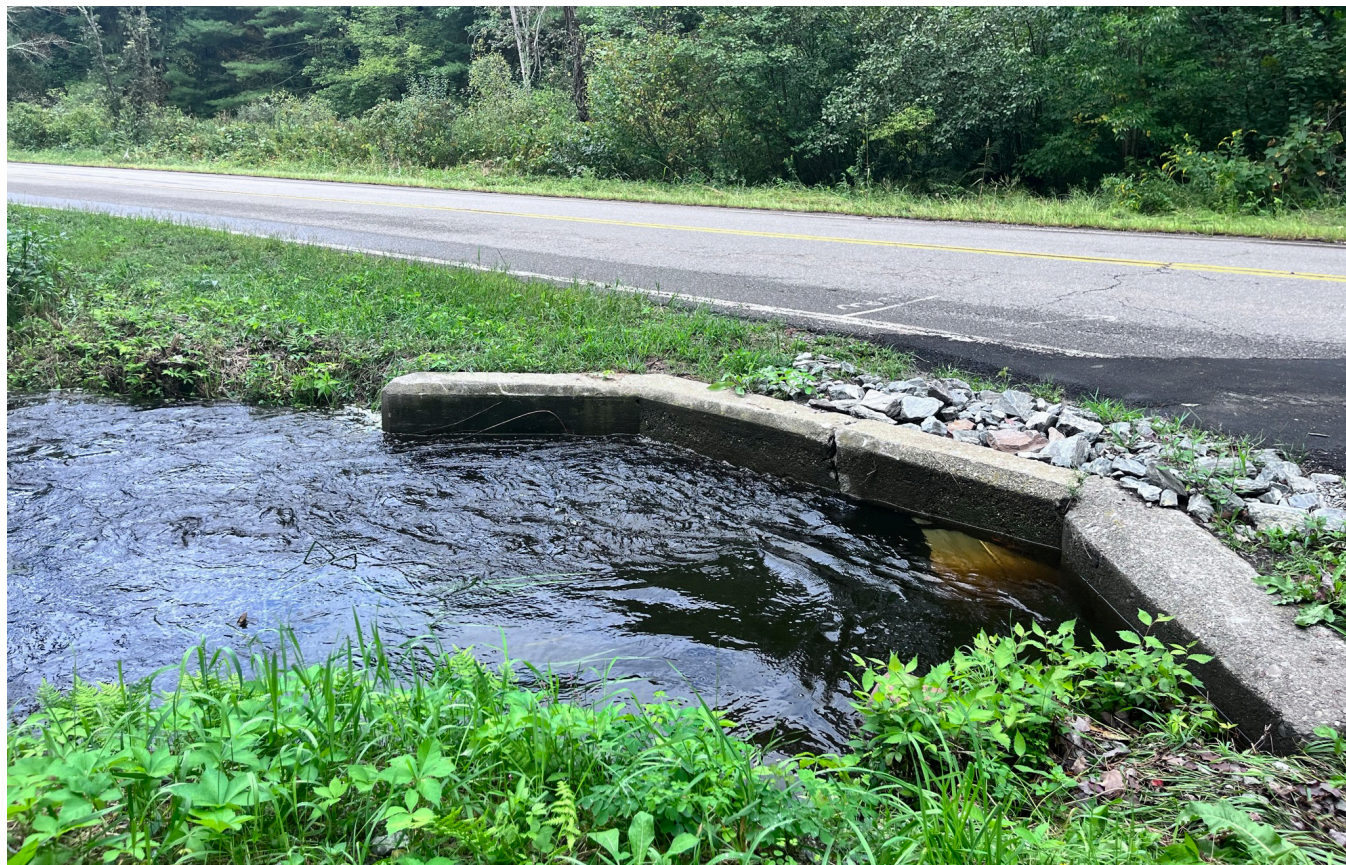
Graphic 3.8.3 Flooded culvert on West Main Street in September 2023. Source: Nitsch Engineering
