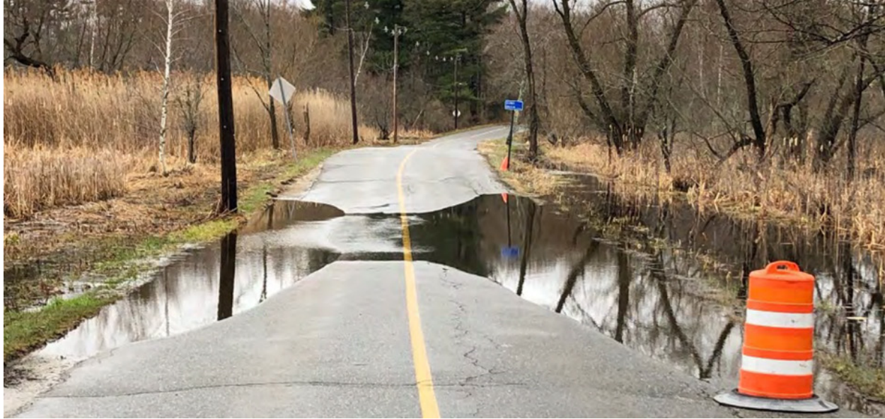
Graphic 3.8.2 Flooding on Broad Meadow Road after a minor rain event in April 2020. Source: Town of Groton 2020 Hazard Mitigation Plan - Municipal Vulnerability Preparedness Plan (2020)
