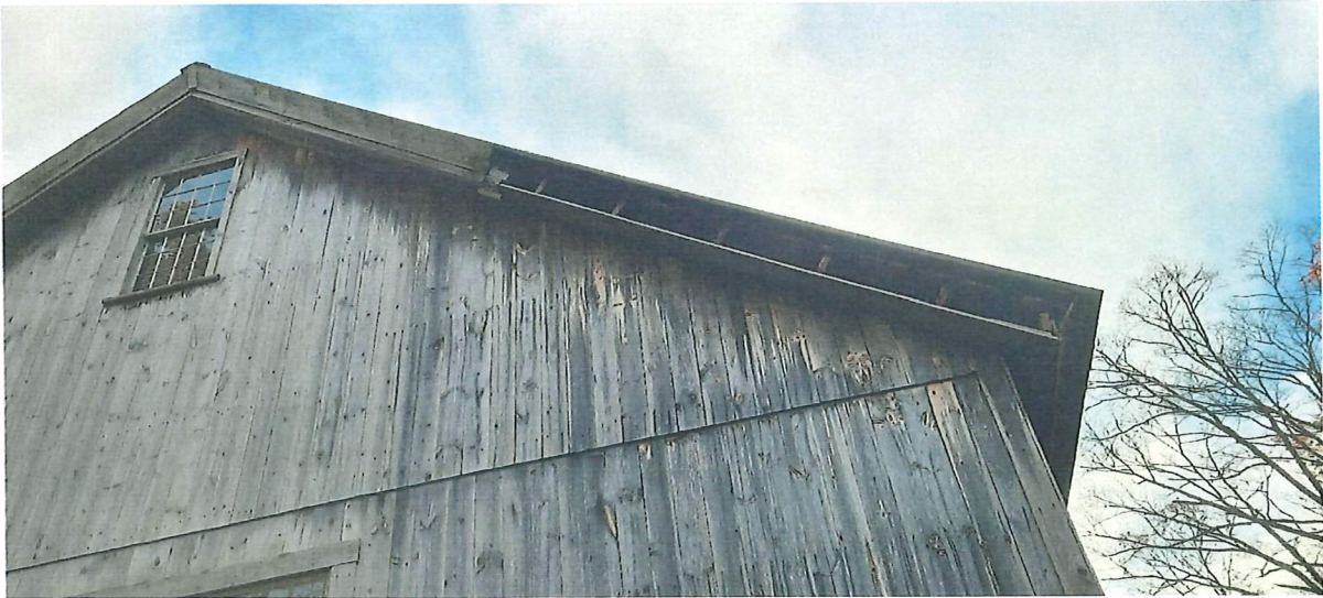
Figure 6: Missing Gable End Fascia from Northeast End of the Barn
