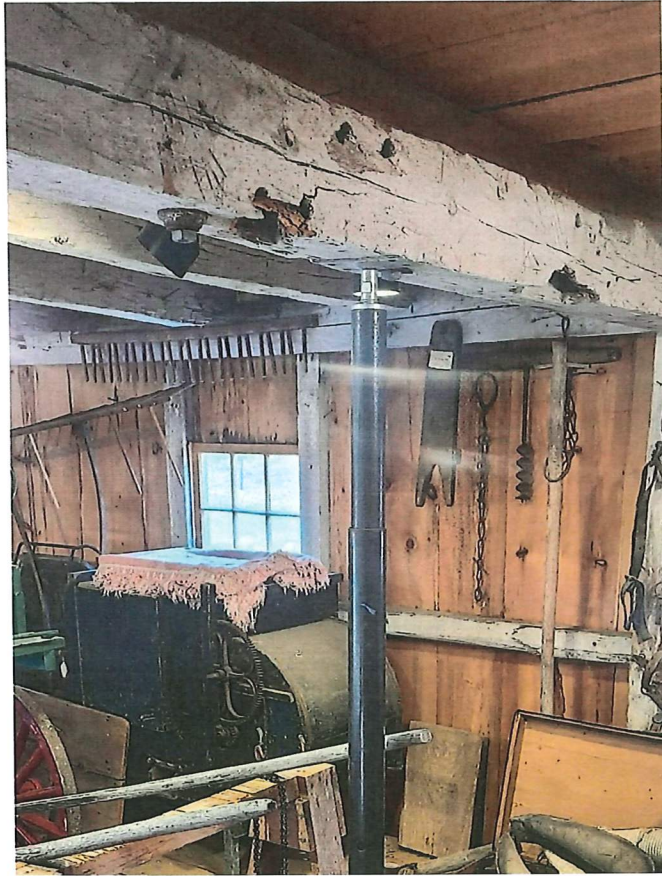
Figure 5: Cracked Beam Under Hayloft with Temporary Stabilizing Jack
