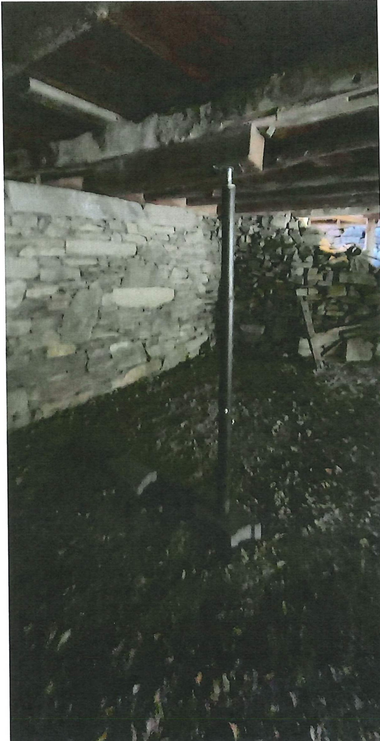
Figure 4: Cracked Main Floor Beam with Installed Stabilizing Jack
